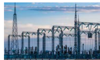
Critical National infrastructure Nuclear
