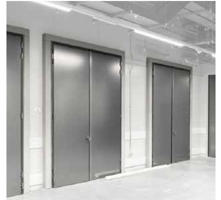
Datacenter / IT room
